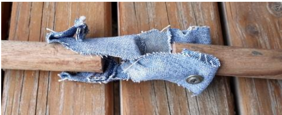
Flexible joint closeup
